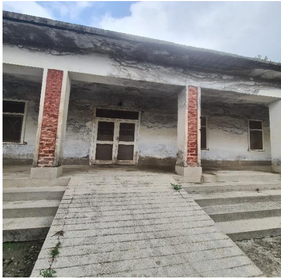
Dental block closed and buiding need repair
